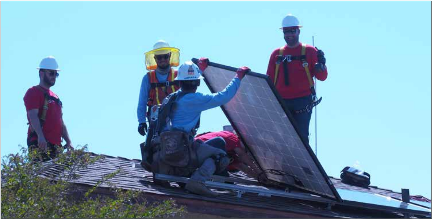
GRID Alternatives LA installing solar panels on a Watts home. Photo credit: Watts Rising
